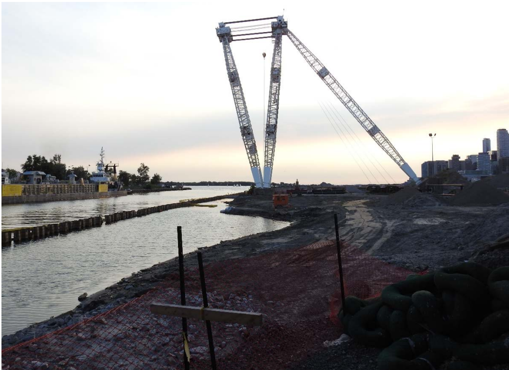
Photo 6 Looking West, at Polson Slip, at what will be the new mouth of the Don, to the Atlas Crane. The crane is being retained as an historic artifact, a reminder of the area's industrial heritage. The foundation base "wraps/shields" are new, to discourage climbers.
