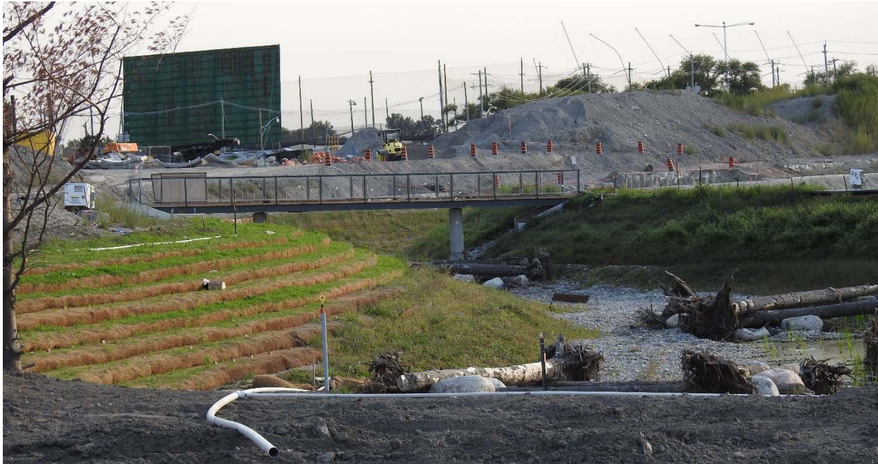
Photo 5 Looking west (roughly) at the new pedestrian bridge across the new river bed
